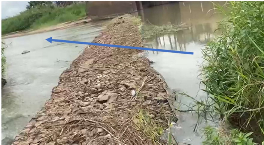
The water diversion weir constructed in year 2022 downstream of the 1H8A flow gauging station, which rendered the existing rating curve useless.
